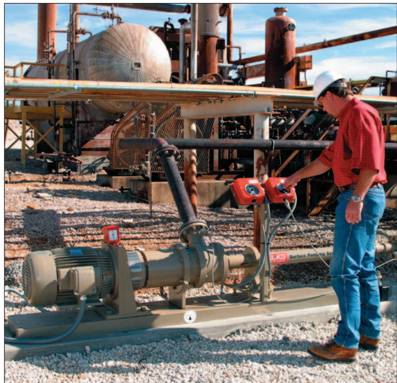
Figure 2. SPS unit in service at a liquid amine facility
