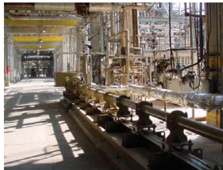
Figure 6. A single surface pump, rated for 160-gpm at 3000-psi with a 400-hp motor, installed in a Louisiana refinery on wash-water pump service.
