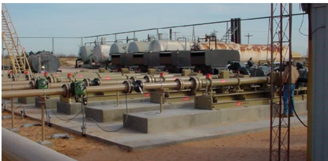
Figure 4. Six surface pumps in West Texas, each rated for 800-gpm at 1600-psi with 800-hp motors used for produced water re-injection.
