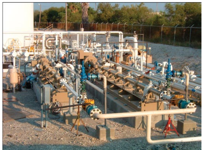
Figure 5. Installation of two surface pumps used to pump methanol to a remote chemical plant via a 4-in pipeline. One pump is rated for 230-gpm at 1100-psi with a 300-hp motor; the other is rated for 330-gpm at 1870-psi with a 450-hp motor.
